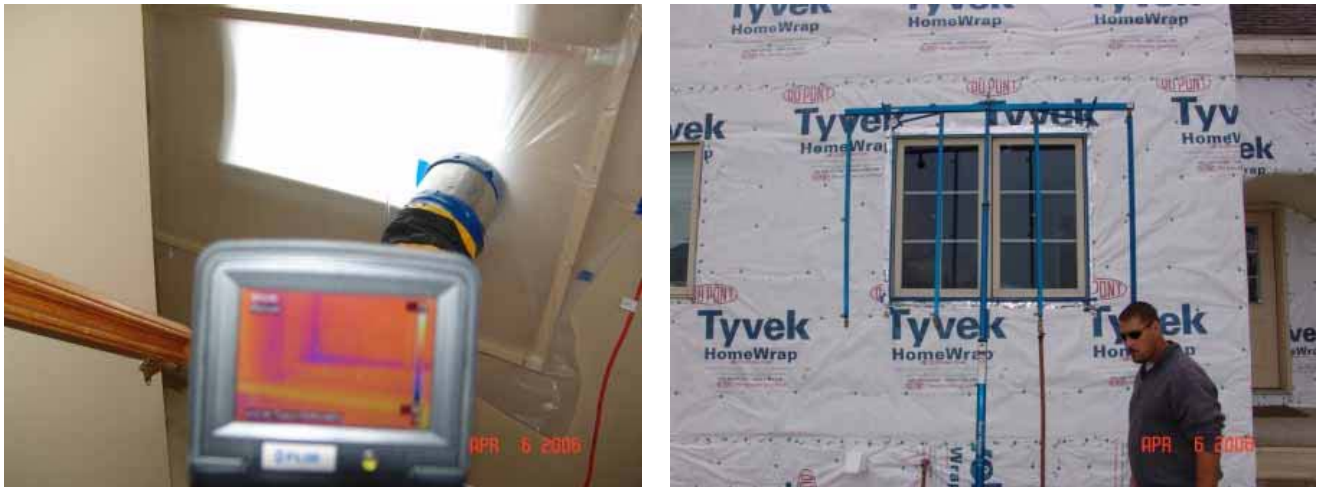
Figure 3. Infrared thermography allows visible access within the testing chamber – Photo of exterior spray rack system
