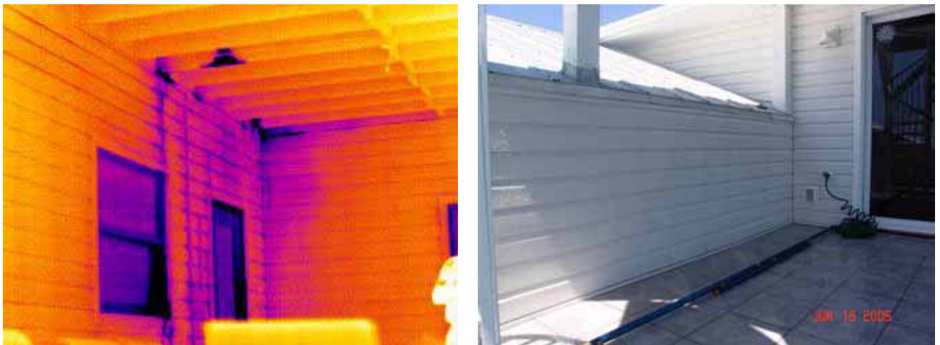
Figure 5. Thermogram/photo showing water migrating behind siding, additional testing found water coming from the above deck.
