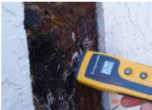
Figure 2. Test cut determined 100% moisture readings using hand held moisture meter.
