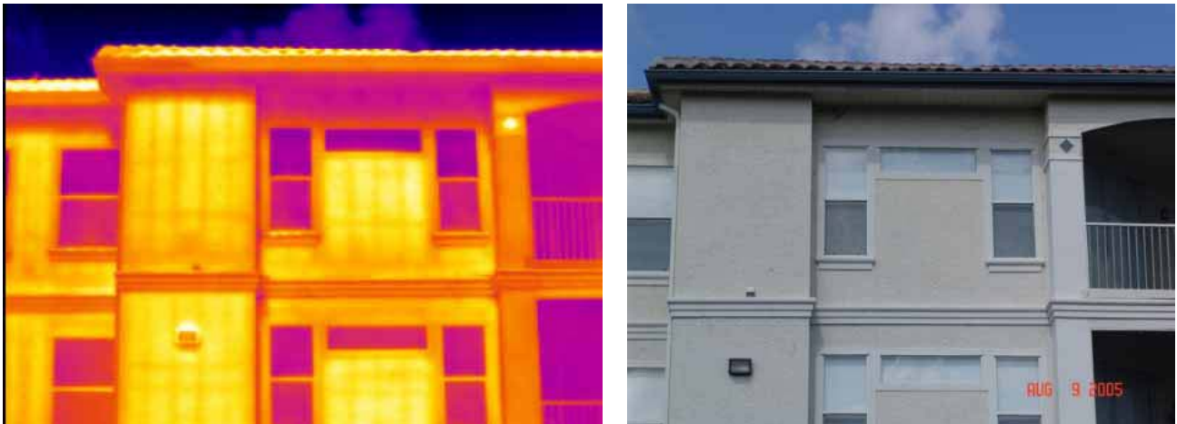
Figure 6. Thermogram/photo showing no anomalies
